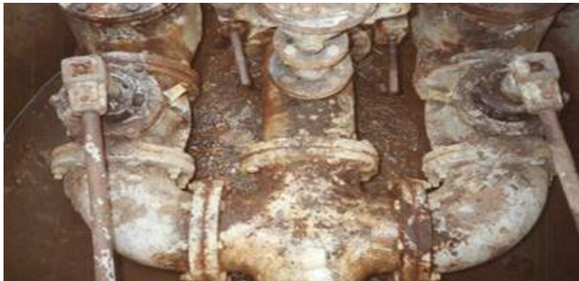
A below ground valve vault in poor condition and not a pleasant or safe place to work.
