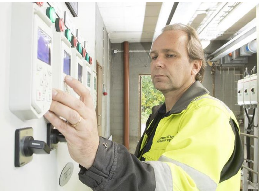
— Water operator using ABB's ACQ580 variable speed drive
